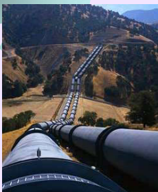
Large diameter pipeline
